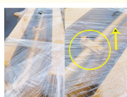
its easy for the pipeline jumps up, causing damage to the pipeline.
